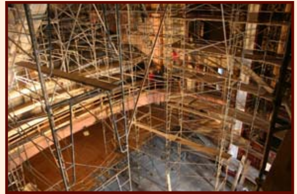
Floor to ceiling scaffolding is erected to facilitate the detailing of finishes
